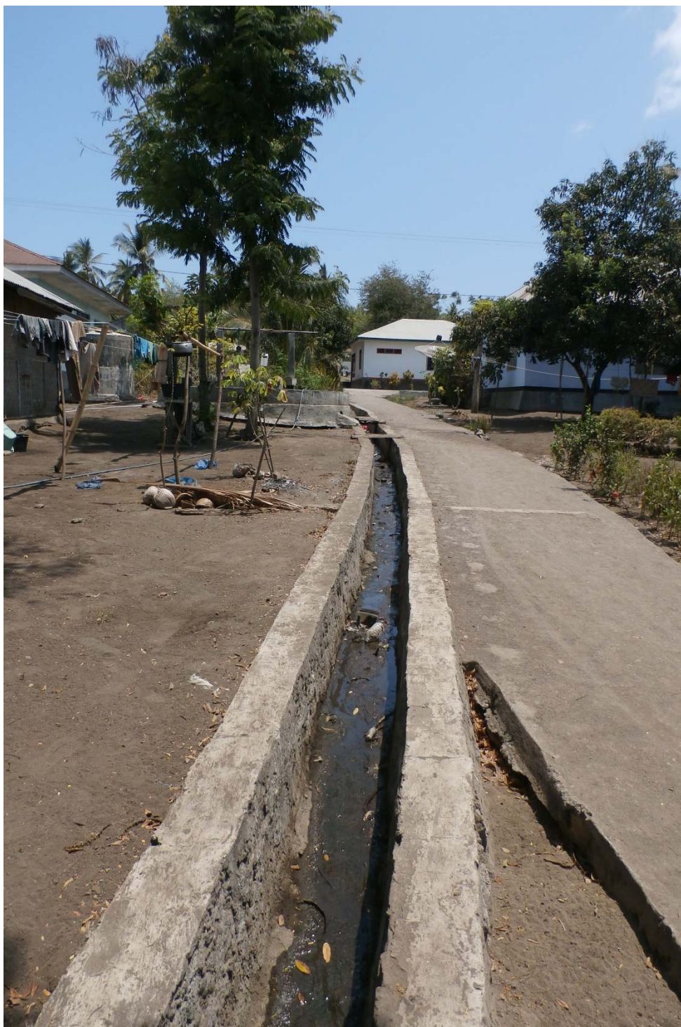
Wastewater is disposed to the ocean
